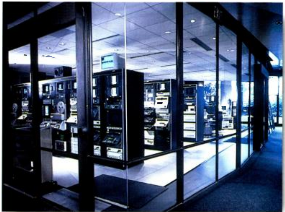
The Post Logic machine room.
